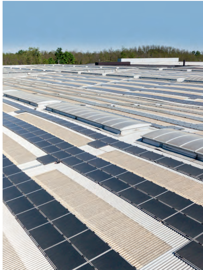
Use of renewable energy
